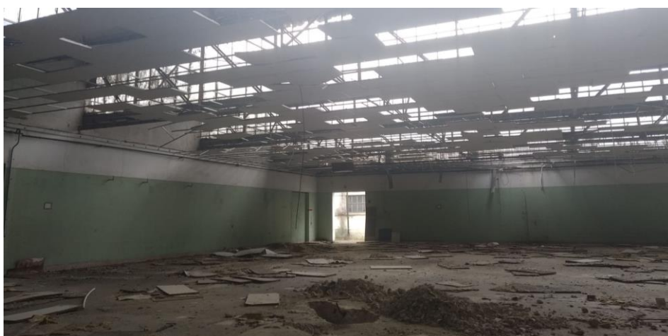
Figure 4. Recent look of the degradation in one of the buildings of the factory (Author Ricardo Triães)
